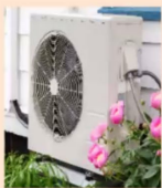
Air Source Heat Pumps
