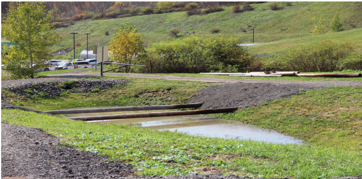
Drainage ditch turned into water trap
