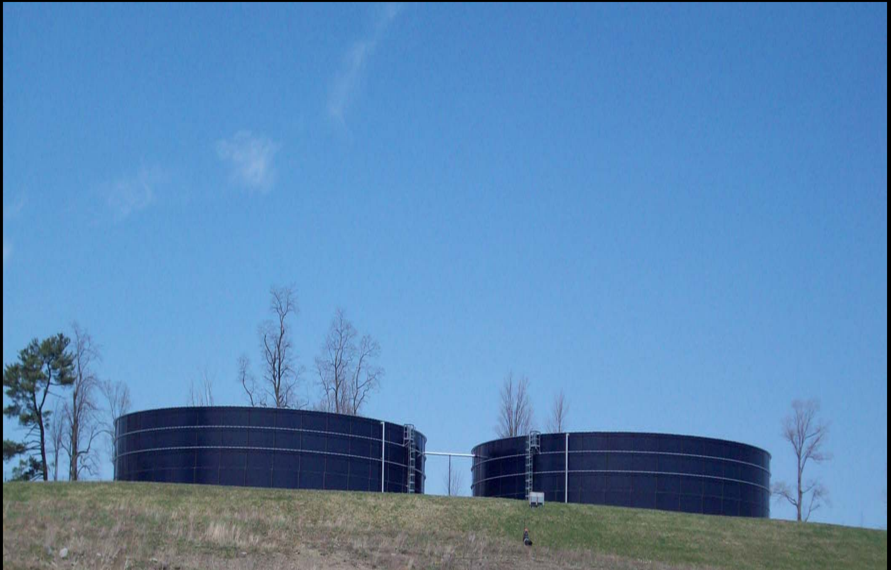
Additional leachate tanks for the new Section IV of the landfill. Each tank can hold 2.2 million gallons of leachate. In August 2009 garbage began to be placed in the new 12 acre cell.
