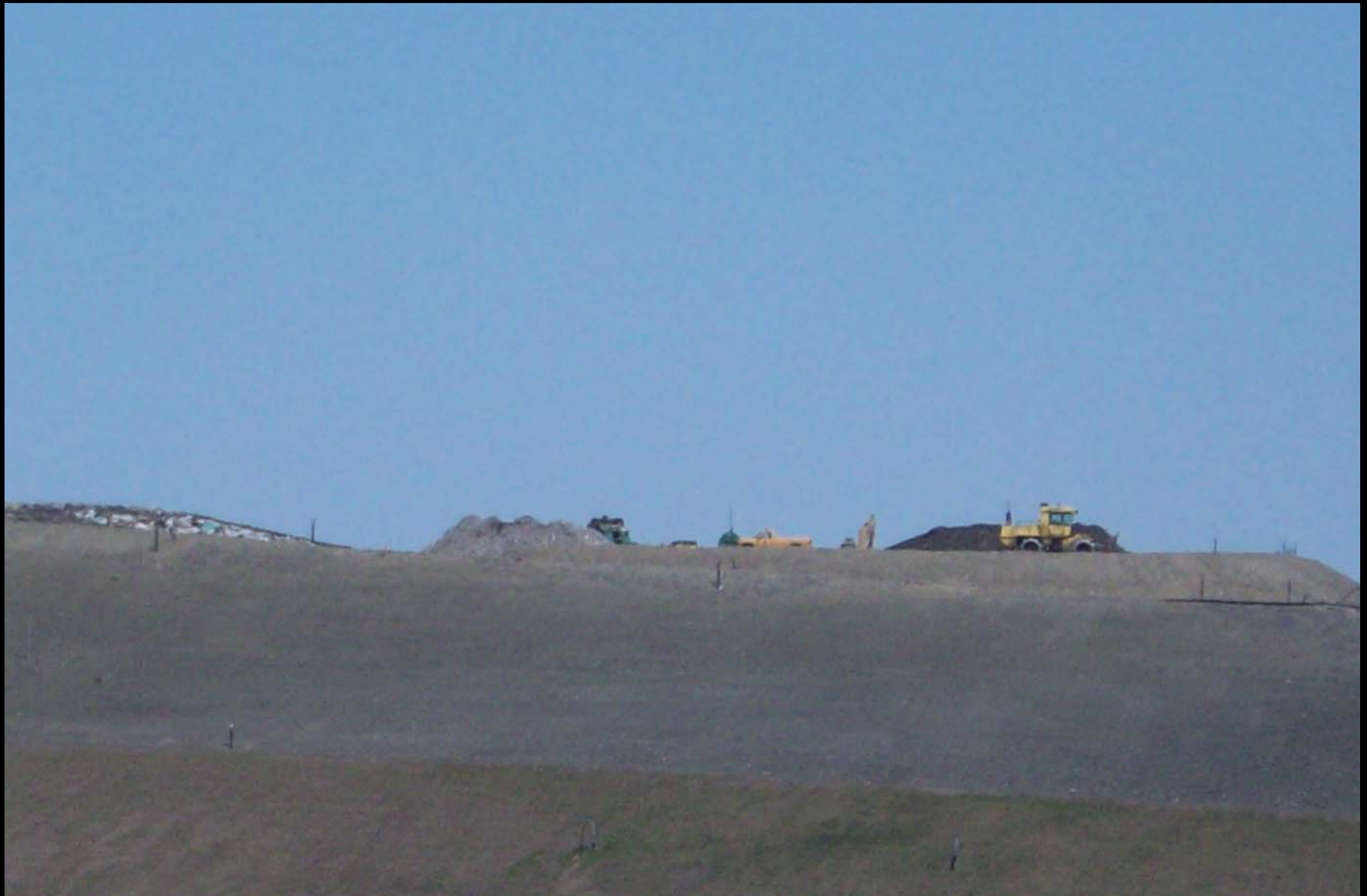
Distant view of the active working face. At the end of each day the garbage must be covered with 6 inches of cover material to keep garbage from blowing and to keep it protected from wildlife.
